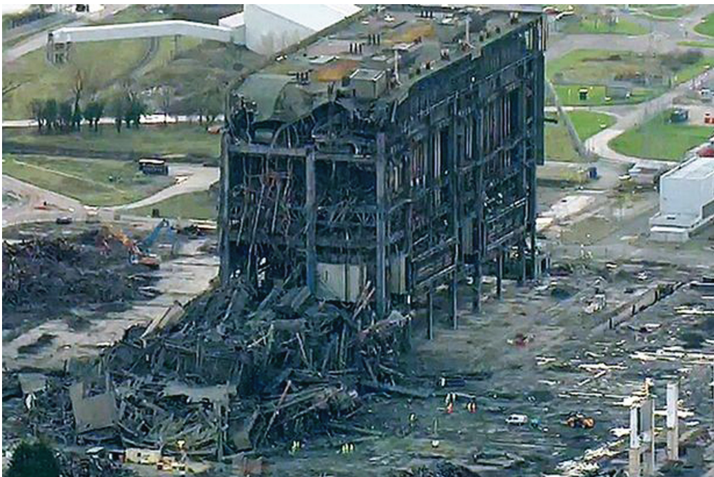
Figure 1: Didcot A power station collapse. UK – 2016 (reproduced with kind permission of PA images)
