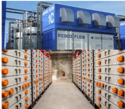
(Flow battery / Lithium Ion )
