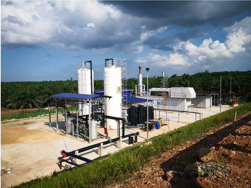
Photo 4. Sri Jelutong Biogas Power Plant in Chini
