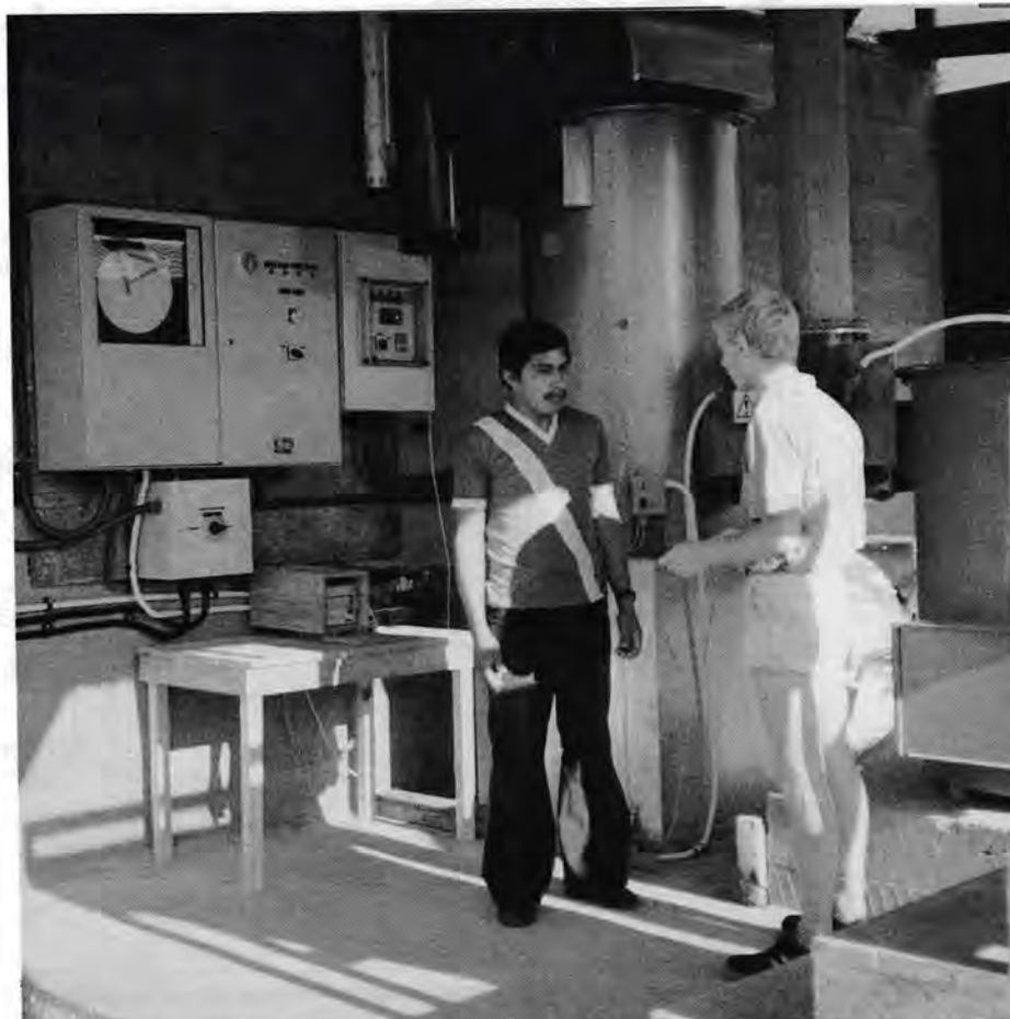
Trainee operator with NRI-designed suspension burner for a timber drying kiln in Belize.
