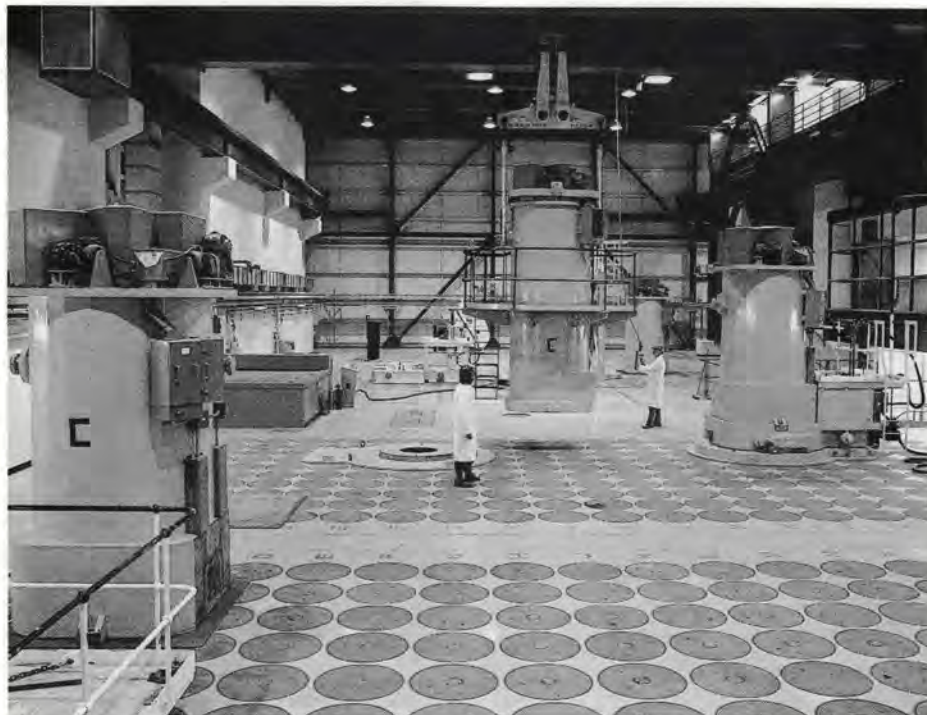
The Vitrified Product Store at Sellafield, built to store containers of highly active vitrified waste cooled by natural air convection.
