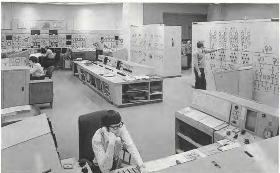
The central control room at the Wylfa Magnox power station, in Gwynedd, the first CEBG power station to use centralised control based on computers. Commissioned in 1972.
