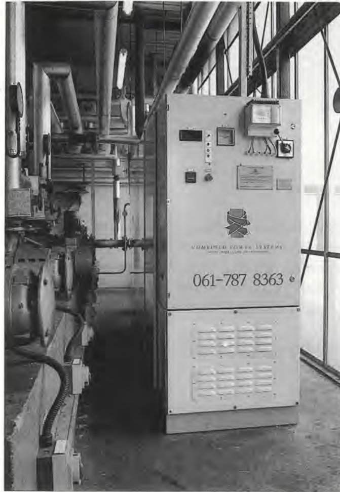
The air fuel ratio controller and catalyst under field trials at Cansfield School, Wigan.
