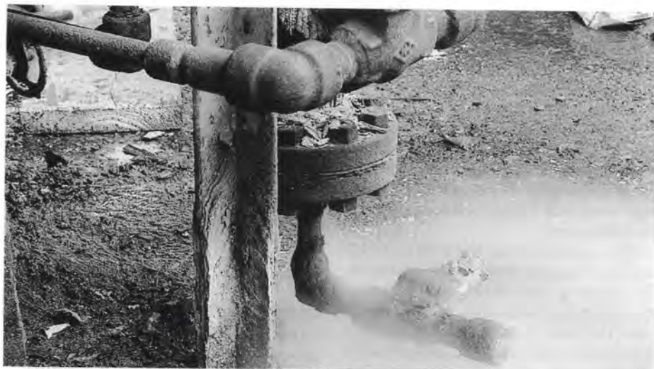
A typical steam leak. Here a flange weld has failed.
