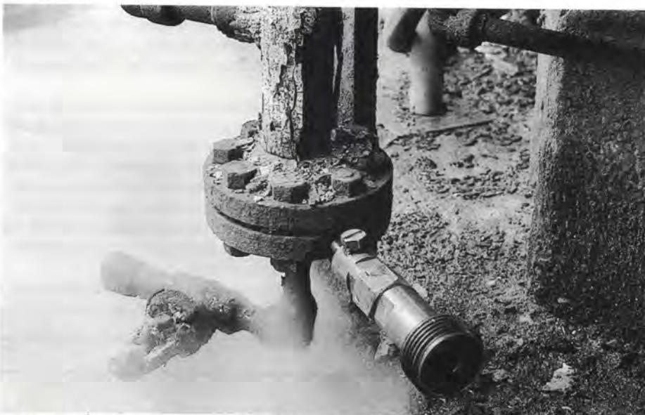
This type of leak can be repaired whilst the plant is on-line. A sealant compound is injected into the flange.
