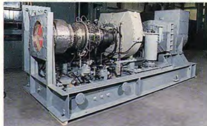
■ 1100kW Dale gas turbine set which now supplies electricity and heat for an Italian brick factory.
