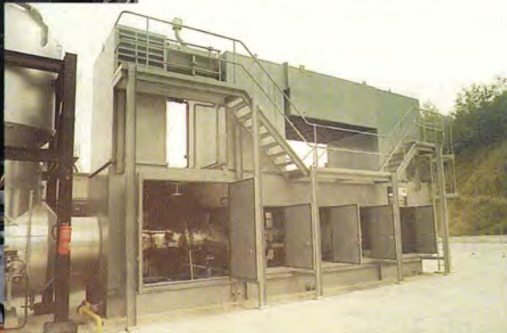
■ This 4.2MW Dale gas turbine set is part of a combined cycle CHP system at a Spanish paper mill.
