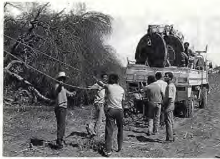
In Ethiopia, manual labour is preferred to machinery: an approach made possible by a large available workforce.
