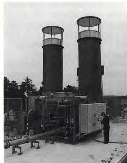
Gas pump set and dual flares at UK Waste's power generation site at Windmill Quarry.
