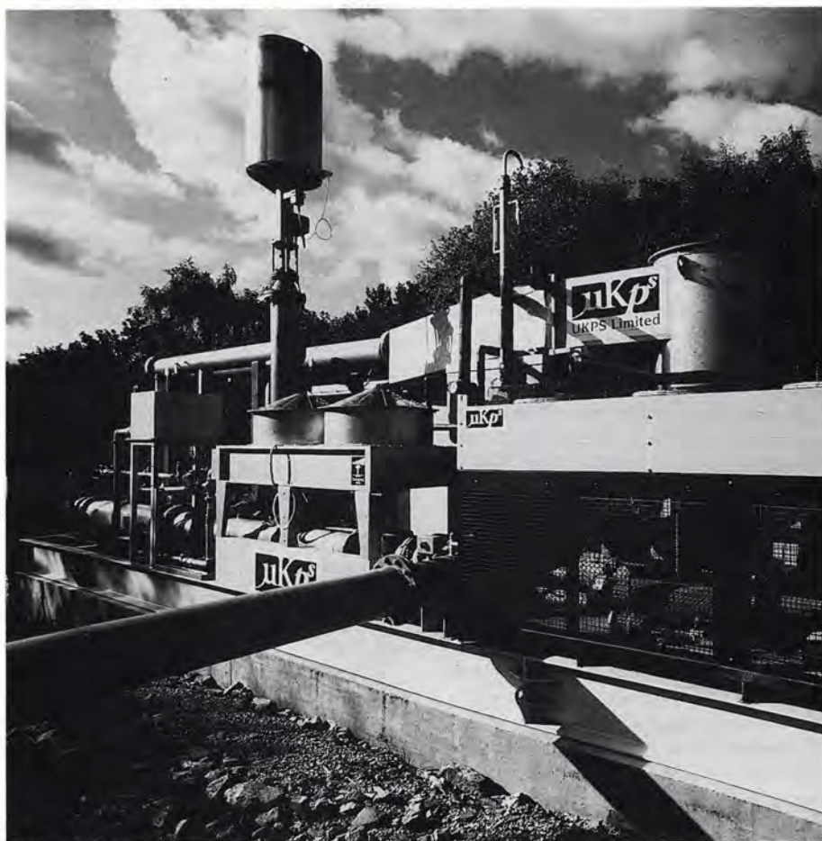
Combined landfill gas flare and chiller plant at Wimpey Energy power station, Appleby Bridge.
