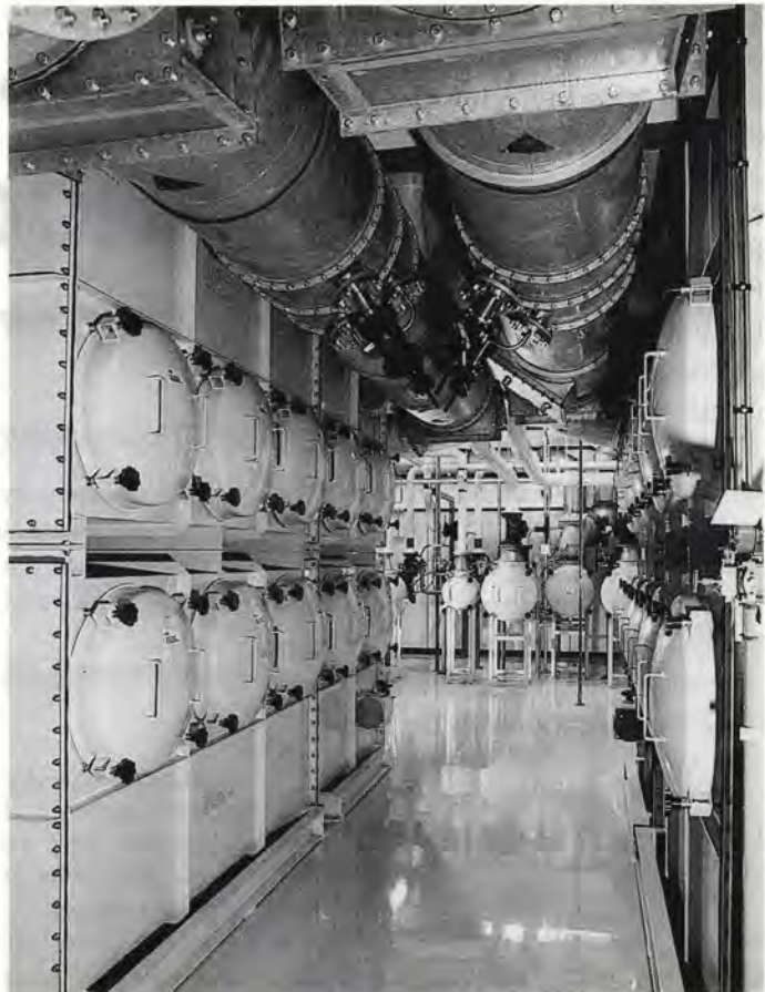
Vokes safe-change filtration system installed at BNFL's new oxide fuels plant. Pictured above is one of the multi-module filtration containment systems installed at Springfields.
