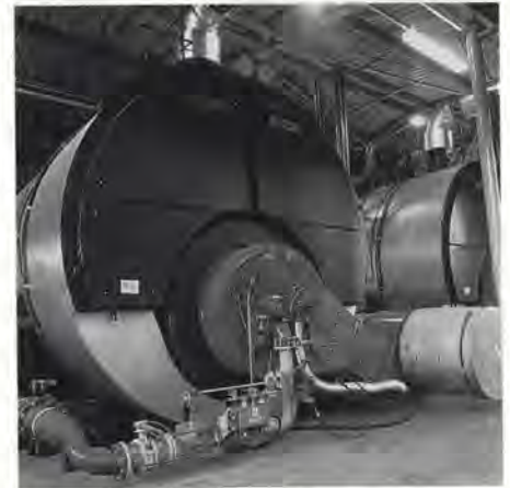
Two 15 MW boilers at the Bernard Road Boilerhouse provide back-up heat for the system
