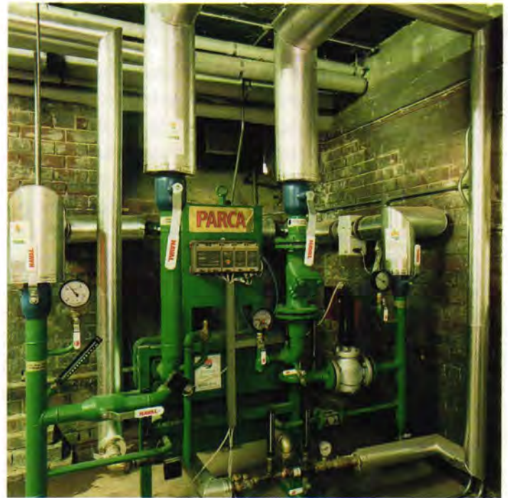
This heat exchanger installation—which replaces boiler plant—illustrates the potential for space-saving with district heating
