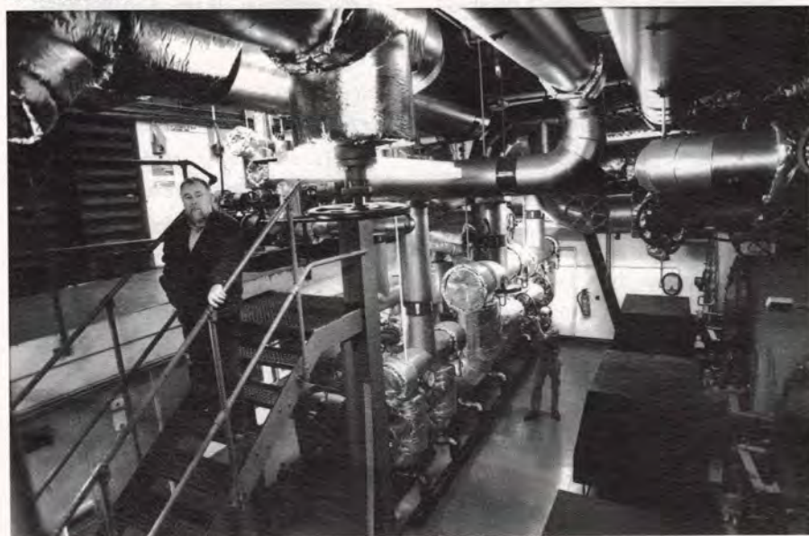
Inside the plant room - a 1 MW CHP unit installed at the Wyndham housing estate in Southwark
