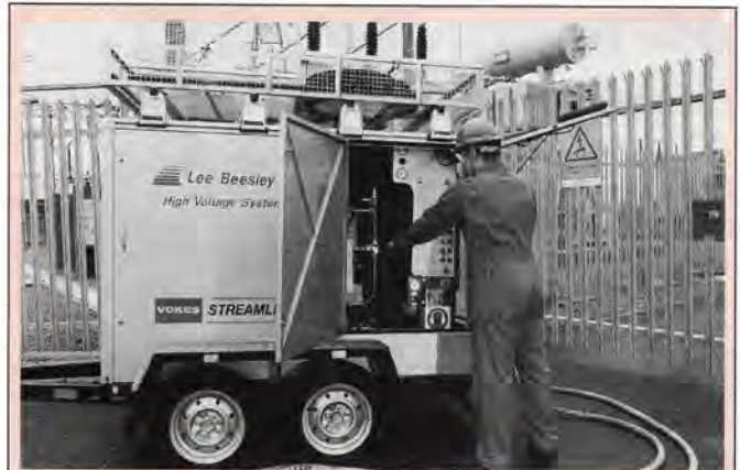
Lee Beesley has introduced a mobile high voltage oil filtration service as part of its portfolio of predictive maintenance programmes. The new on-site service is aimed specifically at high voltage systems users and in particular to assist companies in the development of a transformer maintenance policy.
