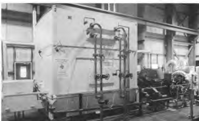
The new steam turbine at Sheffield Heat and Power - now a true CHP operator
