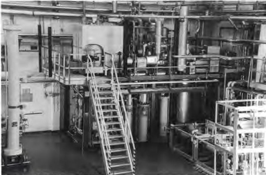
Phosphoric acid fuel cell (PAFC) plant
