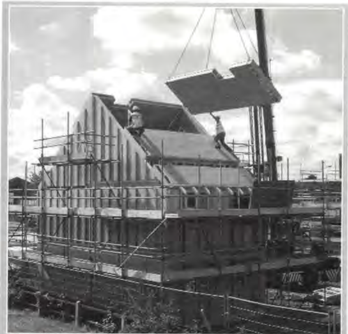
Focus Housing Group scheme at Castle Vale, near Birmingham, demonstrates the potential for the passive approach and the use of prefabrication to improve build quality. The timber frame houses maximise passive solar gain. Passive stack ventilation is used throughout, and a SAP energy rating of 100 was achieved. The prefabricated construction was delivered to site as complete wall panels with the floor and roof in cassette form.
