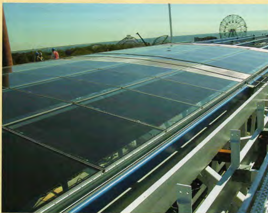
The largest above-ground station on the New York Metro is being renovated to include the installation of a 7000 m 2 roof constructed of RWE Schott solar panels, which will generate around 250 MWh of renewable electricity per year.
