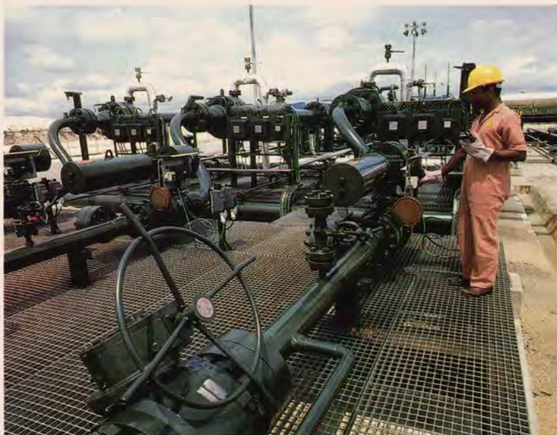
Shell Alakiri gas plant.
