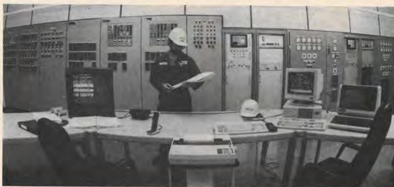
The control room of the power house at Tunnel Refineries.
