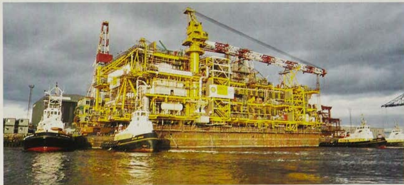
The 9,610 tonne Gannet topside unit being loaded onto a barge prior to being moved downstream to deeper water for final fitout and commissioning. The giant structure had to be moved onto the barge during a narrow weather and tide window which, if missed, could have set the project back several weeks. The final decision for the go-ahead was given at around 4.00 am on the day of the move. The drilling structure, flare tower and accommodation module/helideck will be installed at a later date.
