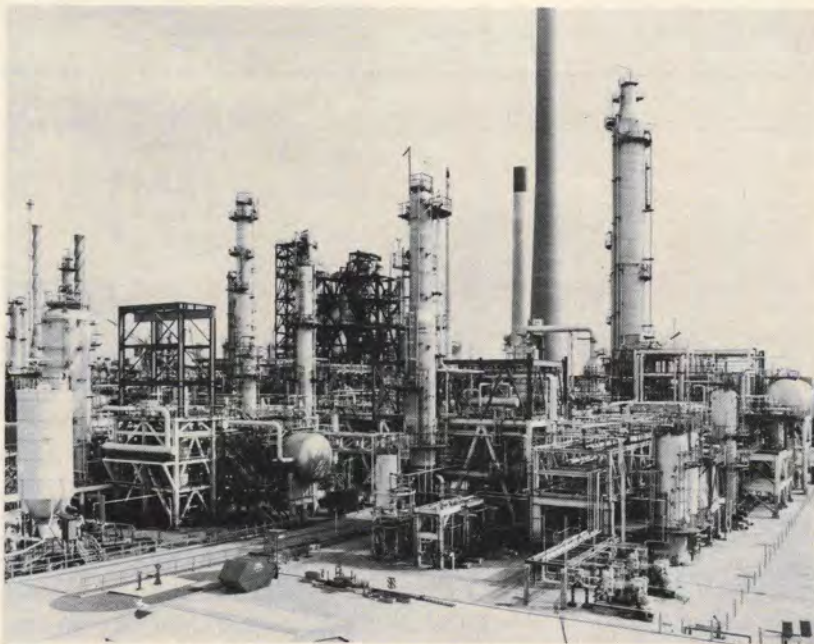
Light ends handling unit constructed using 63 PAUs with a combined weight of 6,000 tonnes.
