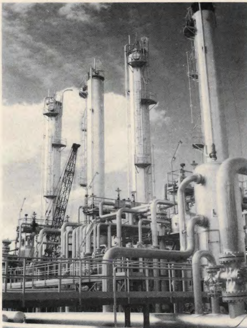
Gas processing plant at Pico Truncado, Santa Cruz Province.
