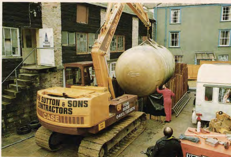
Mr Thompson estimates that seven percent of total development costs are currently being spent underground. 'Oil companies need to make sure they build their sites with the future in mind'.
