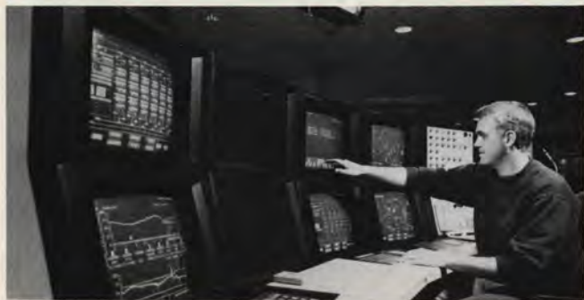
TDC3000 Operator Station in the new Central Control Room.
