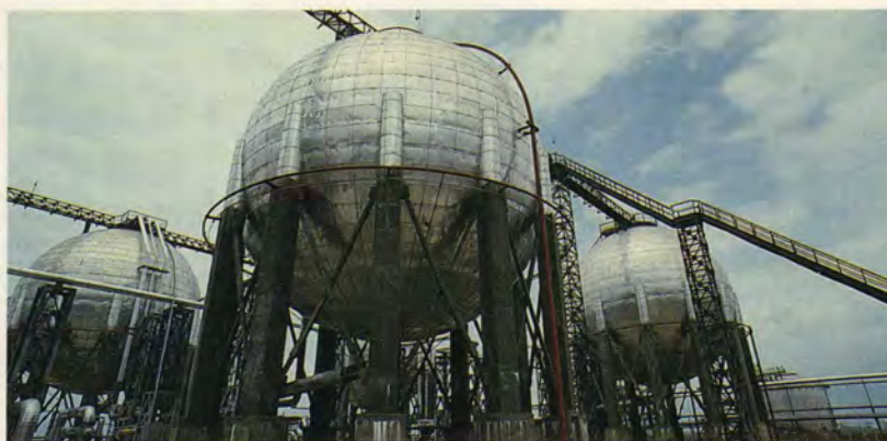
Gas Authority of India's Horton spheres at an LPG extraction plant
