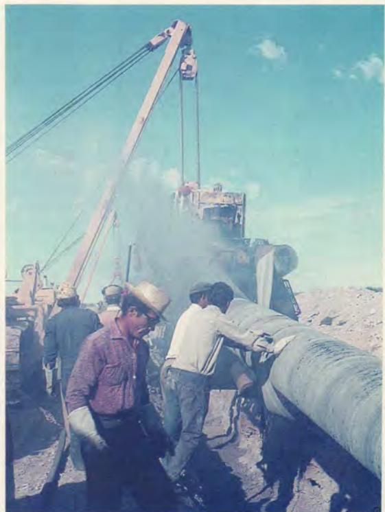
Pipelaying in progress. Chile's nearest source of oil and gas is just a few hundred miles away across the Andes. But dictatorship and border disputes always provided a roadblock
