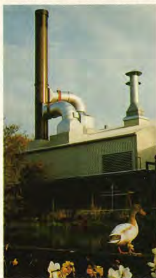
'World's quietest CHP plant'
