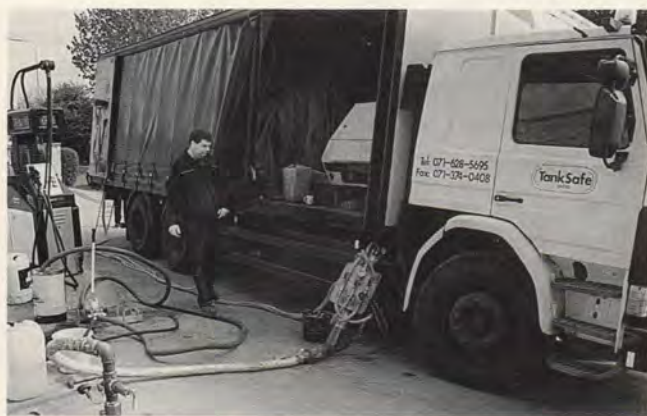
Neutralising storage tanks with foam
