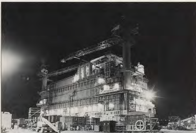
The Heidrun utilities module has been built to last 50 years
