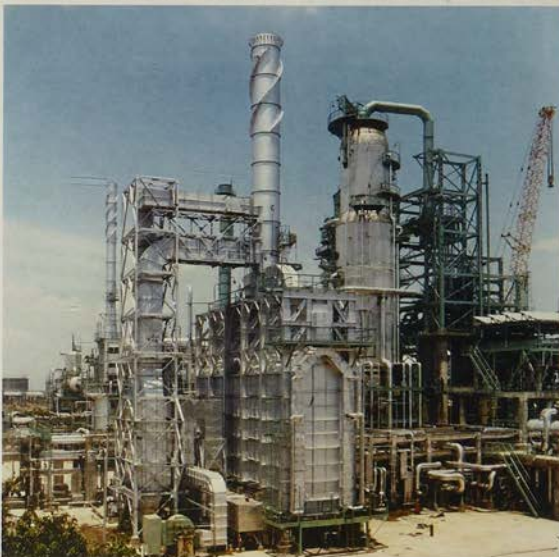
India: Vacuum heater with air pre-heater system
