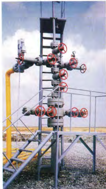
Gas reinjection well in the Dazhangtuo condensate field, part of the Dagang oilfield complex
