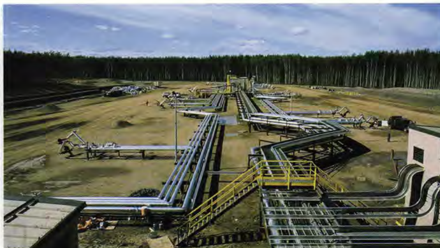
Pipeline network on one of the two current production pads. The pads are located about half a mile from the central plant. MacKay River's 25 initial well pairs are grouped on two such production pads. Pipes carry steam from the central generators to the pads; different pipes carry produced bitumen, gas and fluids back to the plant for separation and processing.
