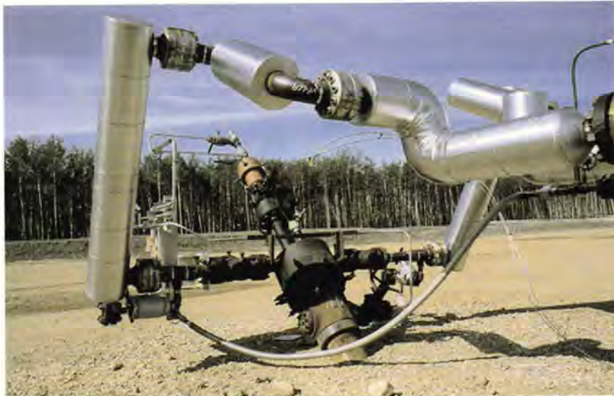
A Mackay River slant production wellhead. A total of 25 wells will be drilled over the field's 25-year lifespan – half of them producers like this one and half injector wells.
