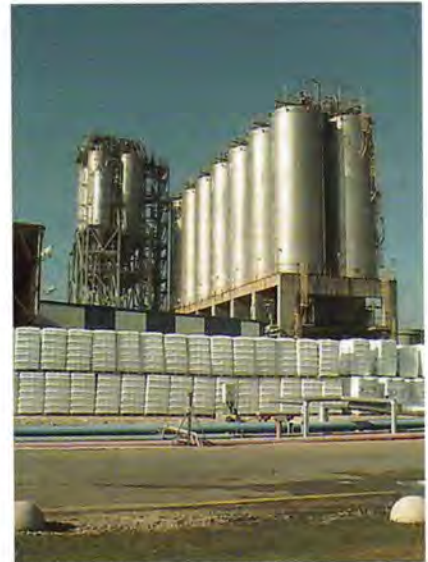
Carmel olefins polyethylene plant near Haifa refinery
