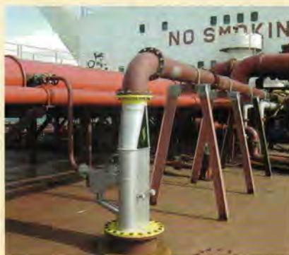
Deckside installation of double venturi static gas compressor. Oil entry at top with side entry of vapour.
