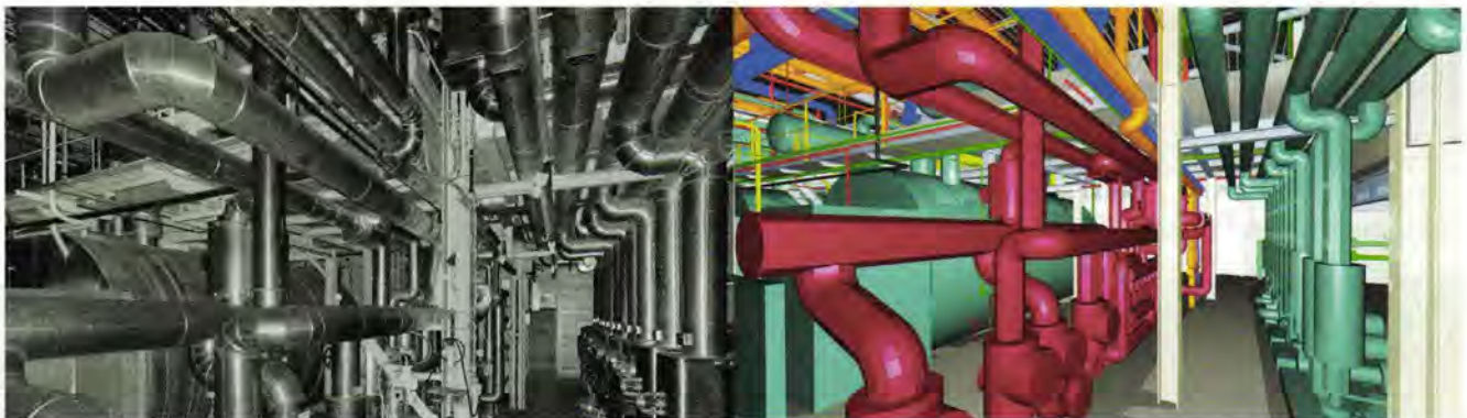
Left: Part of an HVAC system in an automotive plant, showing a number of pipes that have been scanned in a point cloud Right: 3D model derived from scan
