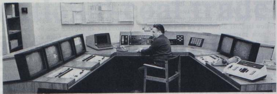
The surface control room at Gascoigne Wood, Yorkshire, where all the coal produced at the £1,050 million Selby mining complex is conveyed to the surface up twin drifts (sloping tunnels) for despatch by rail.
