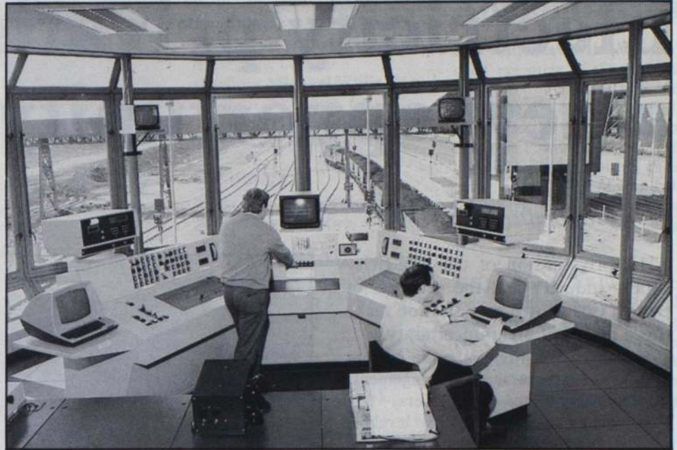
The computerised control centre at the Gascoigne Wood coal handling and despatch plant. The centre controls all the movements of the output of the five mines of the Selby coalfield along a complex series of underground conveyors, through weighing and screening facilities, and manages the movements of the rail wagons which transport the coal off the site to nearby power stations.
