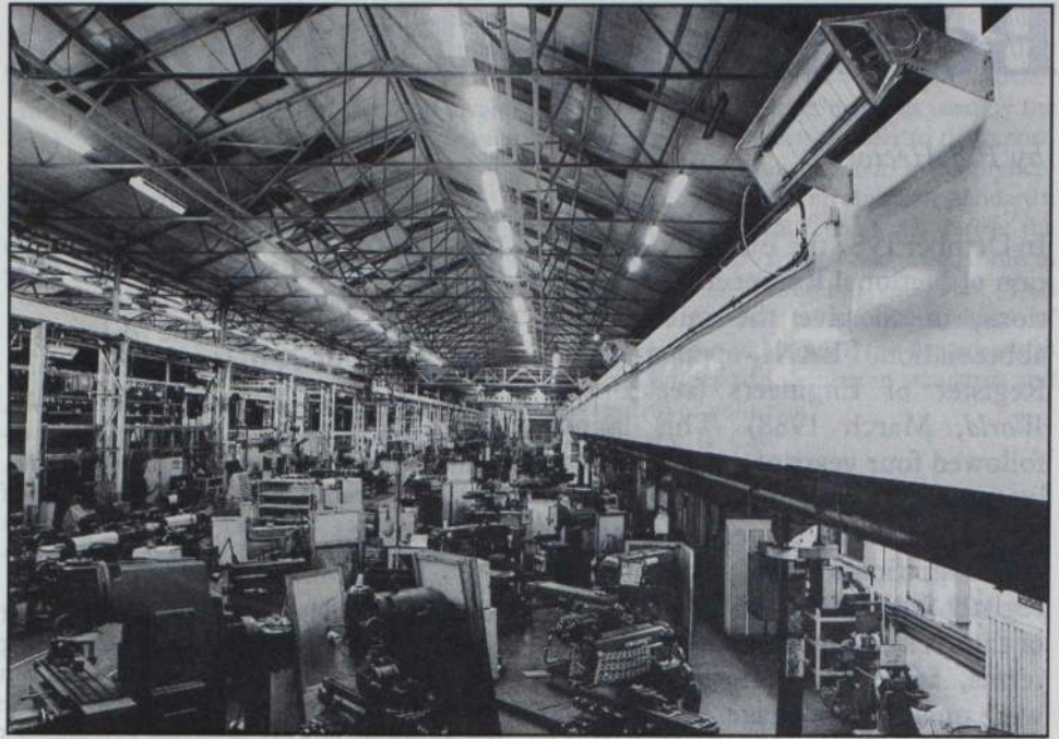
Factory space equipped with a modern, computer-controlled environmental system, which includes heating and air conditioning functions. Such systems are typically saving from 30-50 per cent on previous operating costs.
