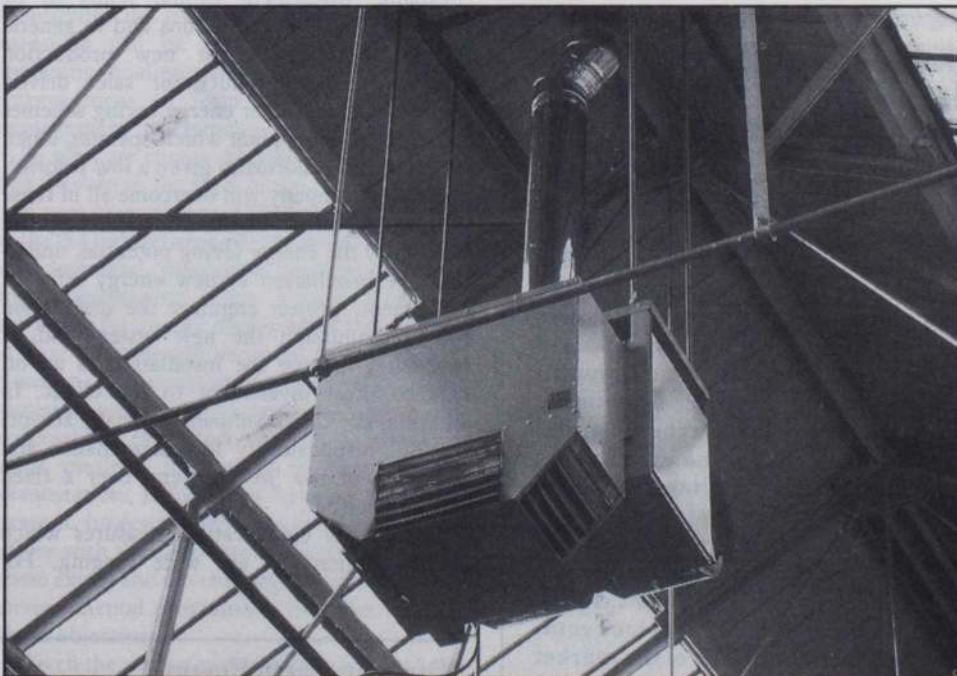
Heating systems designed specifically for each factory have the advantages of low cost and high efficiency plus greater flexibility.
