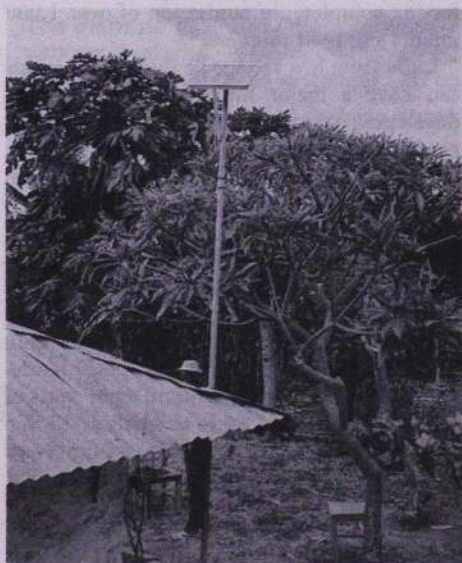
33 Wp photovoltaic panel used for a domestic electricity supply in rural Kenya.
